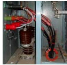
CTF Sensor Install
