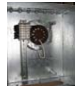
Typical CT junction box
